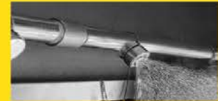
Kitchen Hood Fire Suppression Systems
