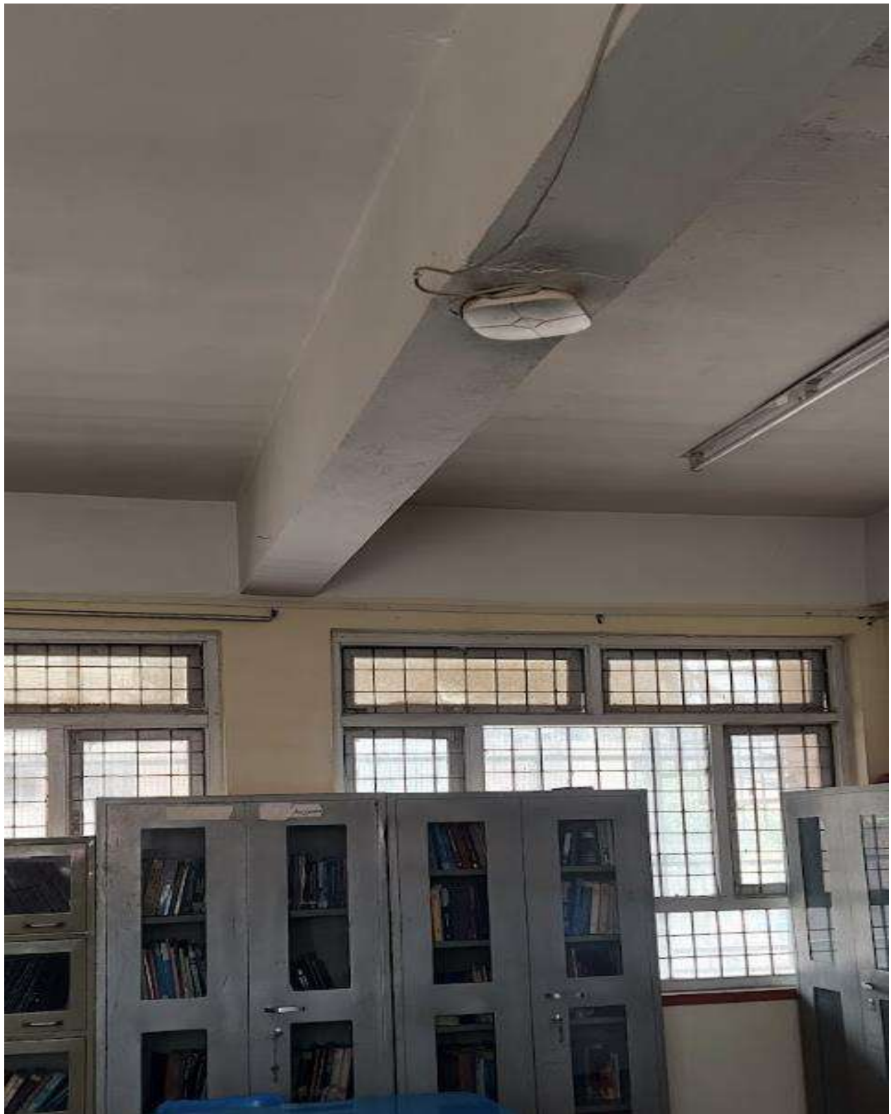
B.5.23.C. Wi-Fi router in library
